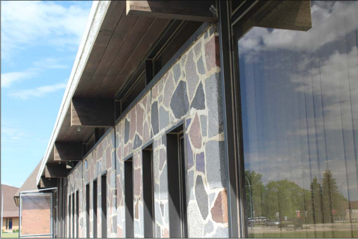
Plate 14 – Windsor Park Library Branch, 955 Cottonwood Road, detail of front (south) façade, 2021. ( M. Peterson, 2021. )
