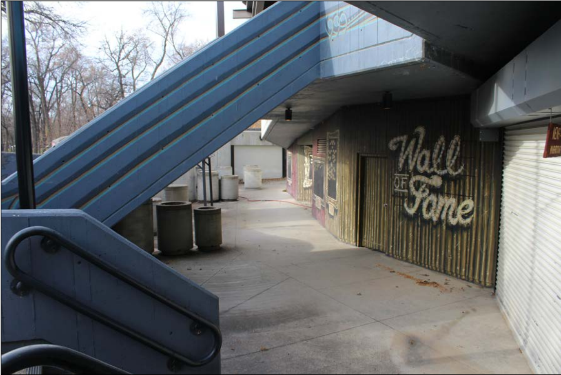
Plate 42 – Main floor entrance area, Rainbow Stage, Kildonan Park, 2015 Main Street, 2022. ( M. Peterson, 2022. )
