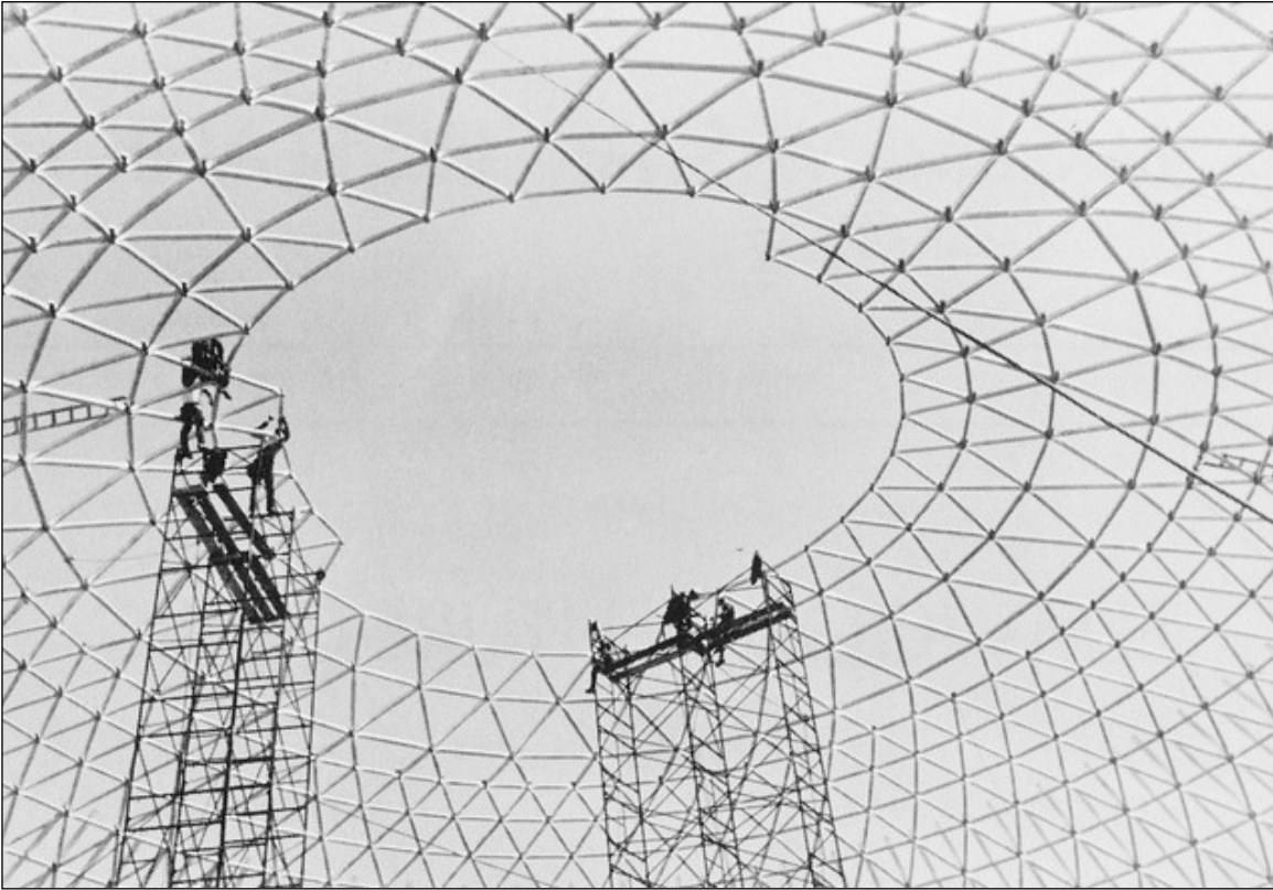
Plate 32 – Construction of the domed roof, Rainbow Stage, Kildonan Park, 2015 Main Street, 1970. ( Photograph by Jerry Olenko. )
